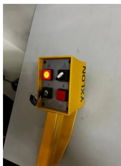
(b) Key in at the control panel
